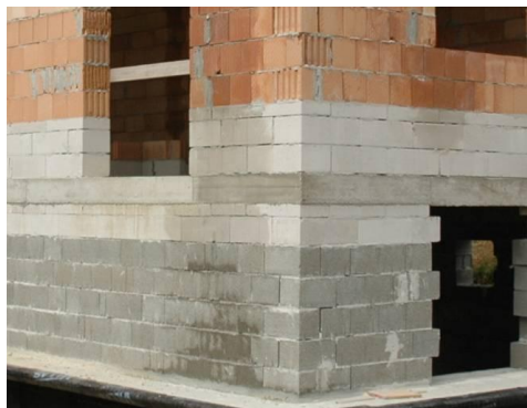
Photo1: even when using clay brick or other materials, AAC can be used to avoid thermal bridges (source: www.passzivhazepito.hu )
